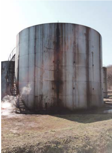
Fig 1. Vertical reservoir / tank
